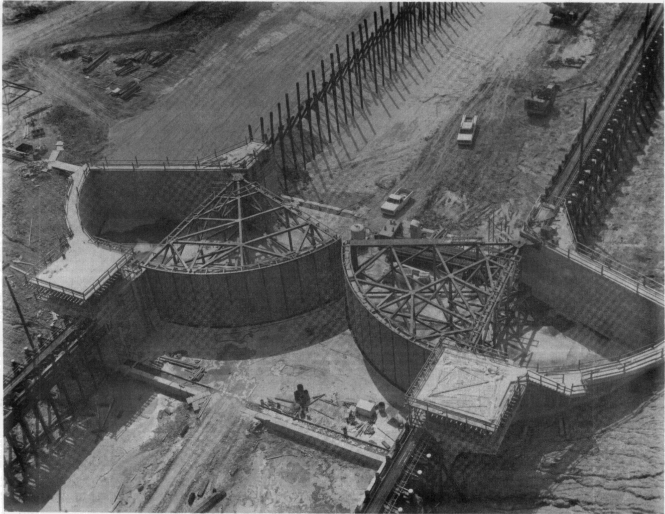
Figure 2-6. Earth embankment with concrete gate bays and sector gates. Vermilion Lock, Gulf Intracoastal Waterway, with design lift = 3 ft (under construction, 1984)
