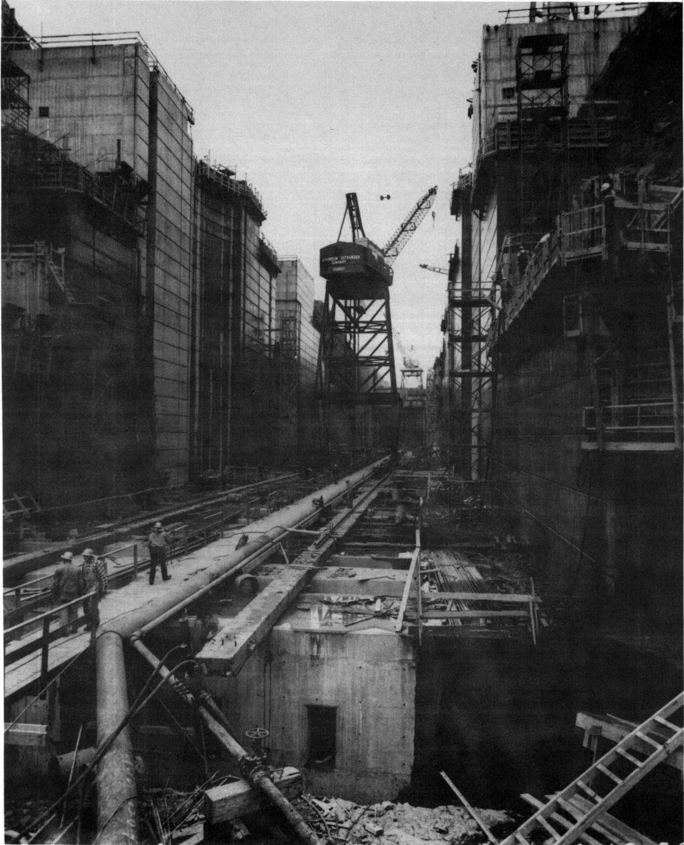
Figure 2-3. Lock with thin walls. The Dalles Lock, Columbia River, with design lift = 88 ft (under construction)
